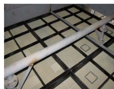
Figure 1.68: Example of a module position used for the SCR technique Source: [140, Italy, 2007]
