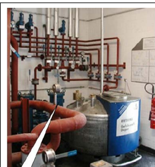
Figure 6.27: Pumping station number 2 with a filter and a waste container for cleaning the filter
