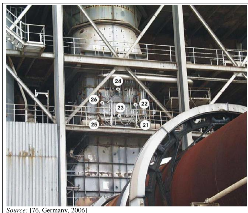
Figure 6.8: High efficiency SNCR and place for injection of ammonia water via lances at places Nr. 21 to 26
