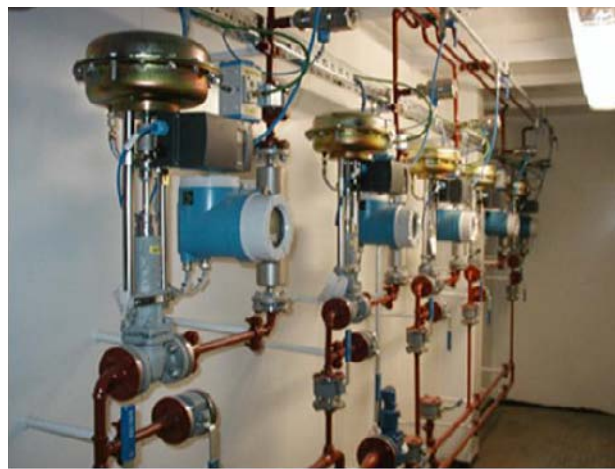
Figure 6.28: Measuring and dosing station with pneumatic valves
