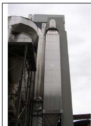
Figure 1.66: Example of an SCR installation Source: [140, Italy, 2007]
