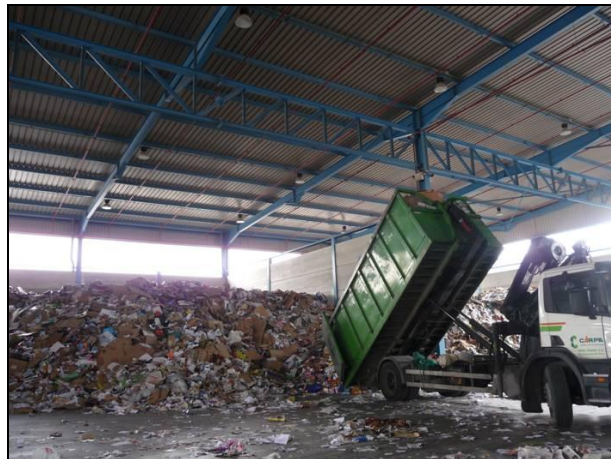
Figure 6.29: Unloading and storage of loose paper for recycling in an enclosed facility with a roof
