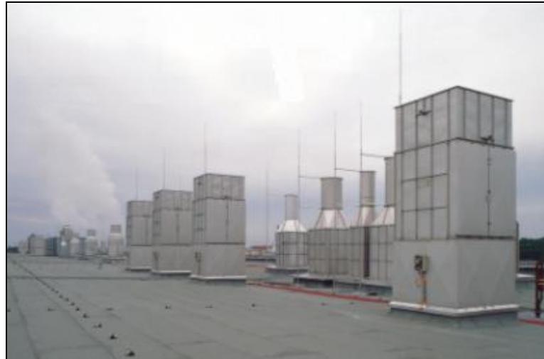
Figure 7.37: Silencers on the paper mill roof
