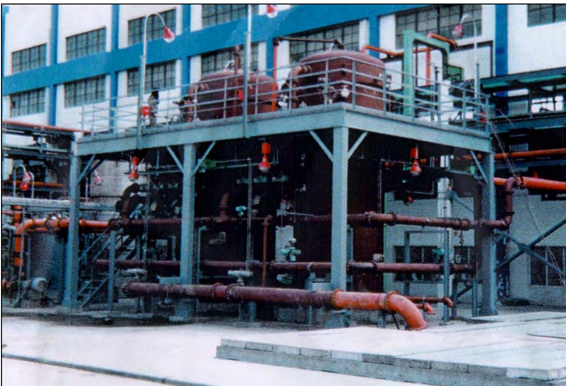
Figure 2.13: View of polishing filters in a secondary brine purification system (photograph supplied by Asahi Glass Co)
