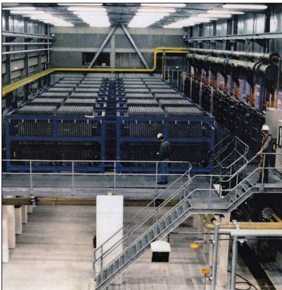
Figure 2.10: View of a membrane cell room equipped with bipolar electrolyzers (Source: Hoechst-Uhde)
