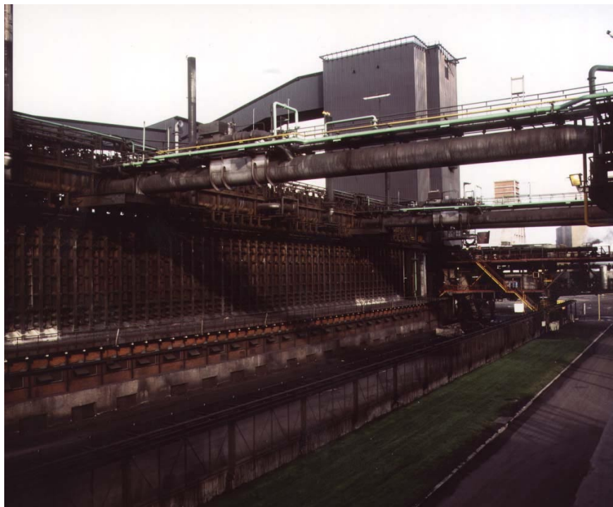
Figure 6.1 : Photograph of a coke oven battery showing the chambers, the coal tower and the coke oven gas collecting main
