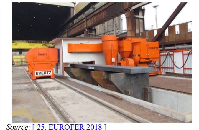
Figure 2.75: Grinding machine equipped with waste gas cleaning abatement system at Tata Steel IJmuiden
