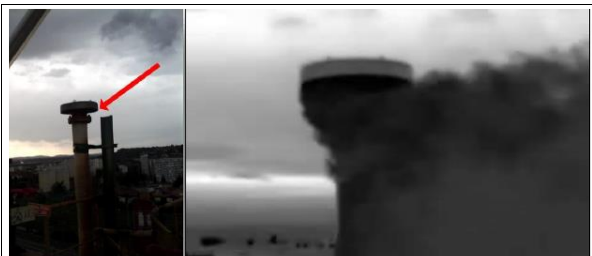
Leak on vent
