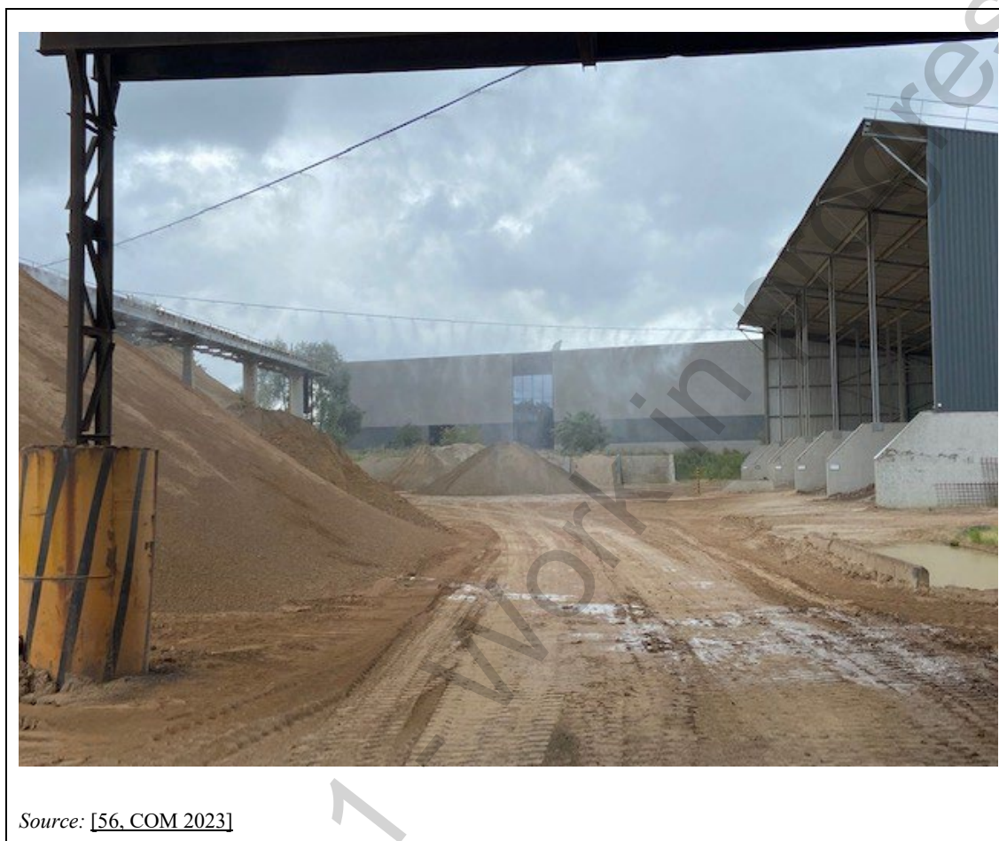
Figure 4-15: Example of a water sprays to reduce diffuse emissions in storage areas
